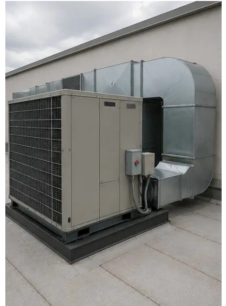
Photo #11. HVAC equipment condition assessed
