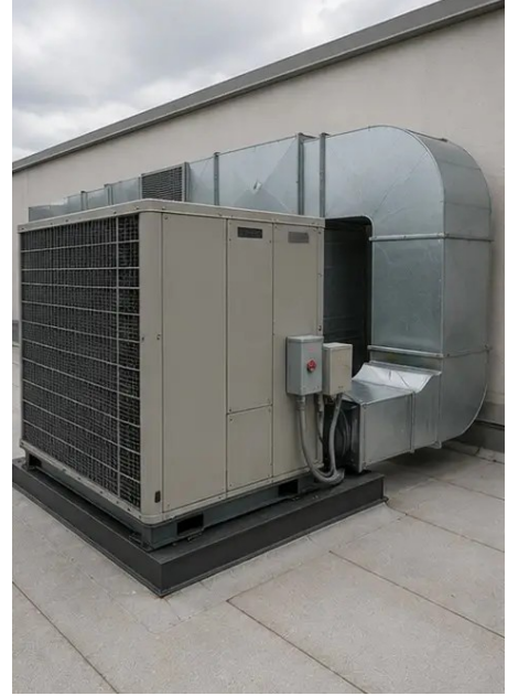
Photo #11. HVAC equipment condition assessed
