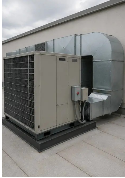
Photo #11. HVAC equipment condition assessed
