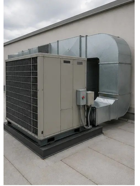
Photo #11. HVAC equipment condition assessed
