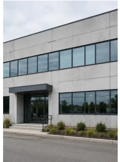
Photo #2. Framsidans fasadskick under besiktning
