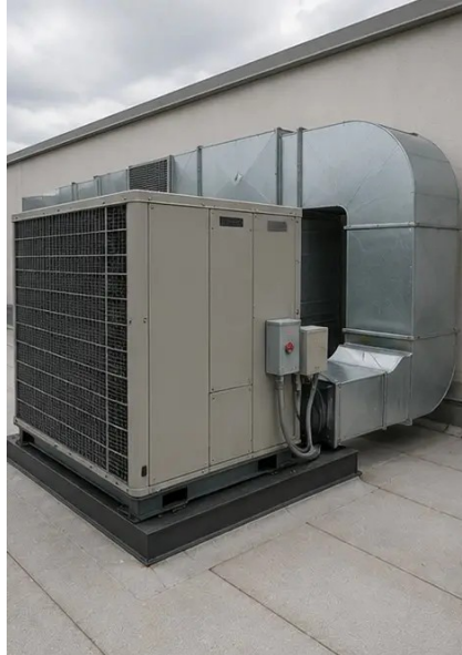
Photo #11. HVAC equipment condition assessed
