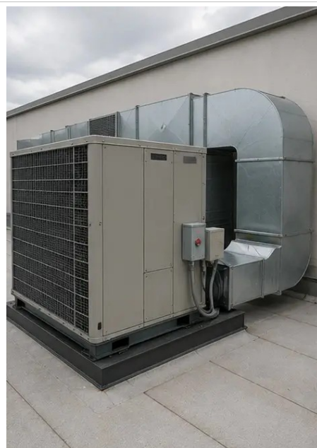
Photo #11. HVAC equipment condition assessed
