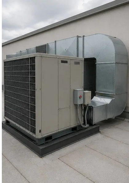
Photo #11. HVAC equipment condition assessed
