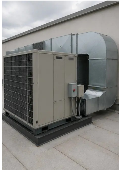
Photo #11. HVAC equipment condition assessed
