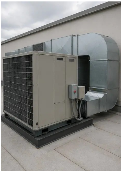
Photo #11. HVAC equipment condition assessed
