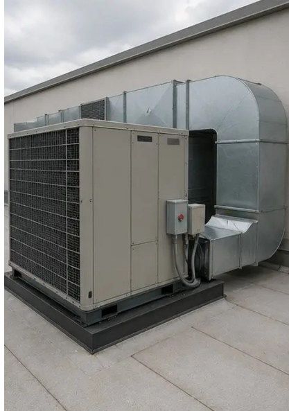
Photo #11. HVAC equipment condition assessed
