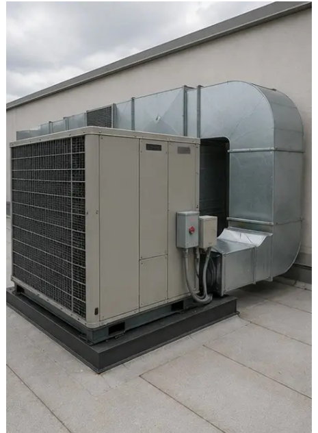
Photo #11. HVAC equipment condition assessed
