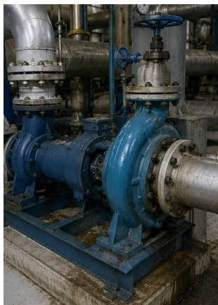
Photo #3. Industrial pump condition assessed during maintenance
