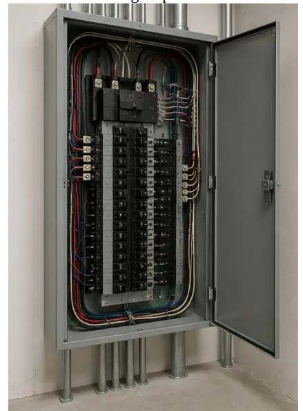
Photo #9. Electrical panel condition documented
