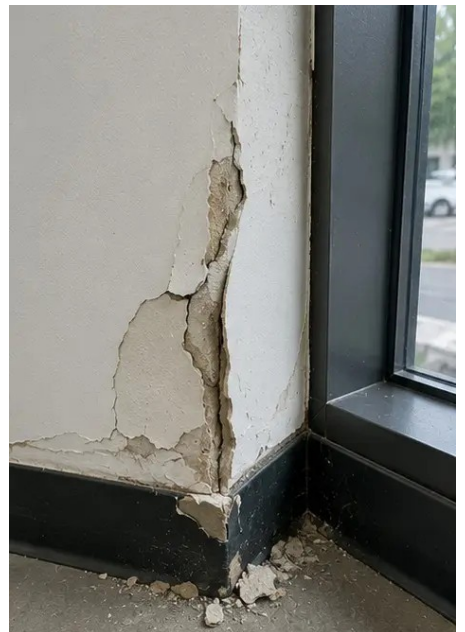
Photo #15. Identified defect area documented for further evaluation
