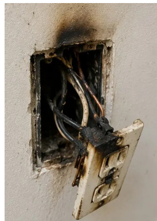
Photo #12. Electrical system damage recorded during inspection
