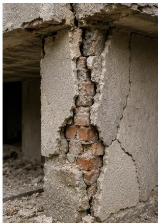
Photo #13. Structural damage detail documented for assessment
