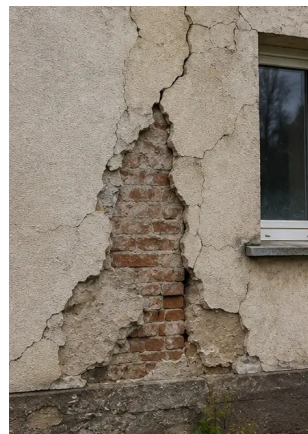
Photo #4. Exterior wall damage documented for assessment
