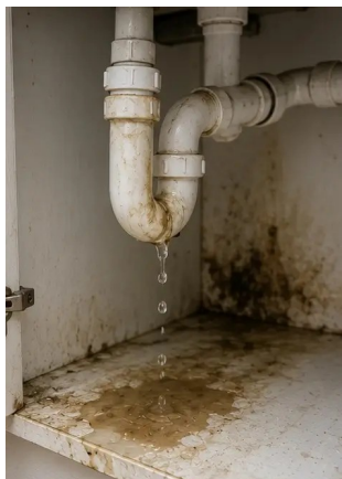
Photo #11. Plumbing leak damage documented
