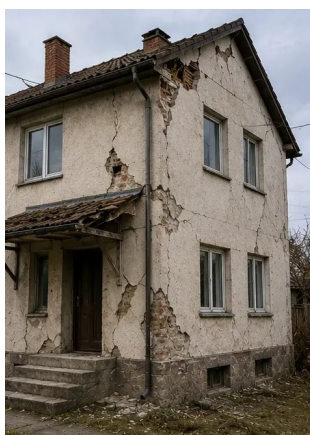
Photo #15. Overview of multiple damage locations
