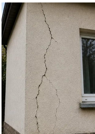
Photo #5. Structural wall crack documented during inspection
