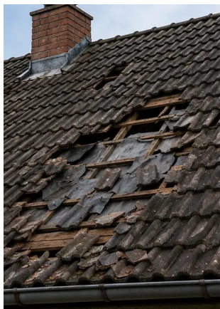
Photo #3. Damaged roof area identified and recorded
