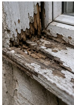
Photo #14. Close up evidence photograph of identified damage
