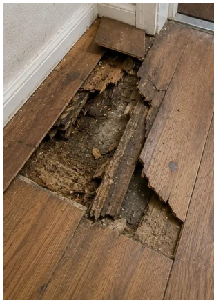
Photo #9. Damaged flooring documented during inspection
