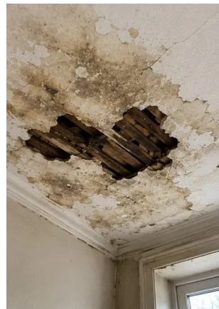
Photo #10. Ceiling damage identified and recorded
