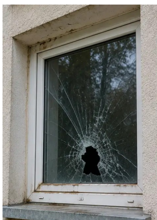
Photo #7. Damaged window documented for evaluation
