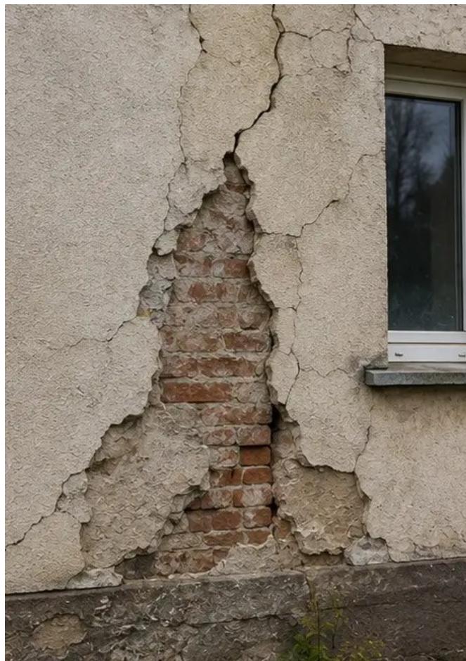
Photo #4 Exterior wall damage documented for assessment
