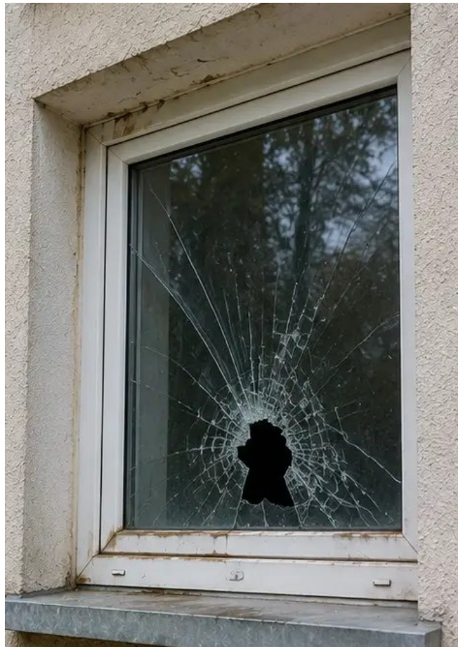
Photo #7 Damaged window documented for evaluation
