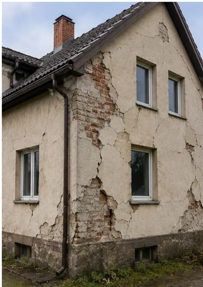
Photo #2 Exterior damage overview documented during inspection
