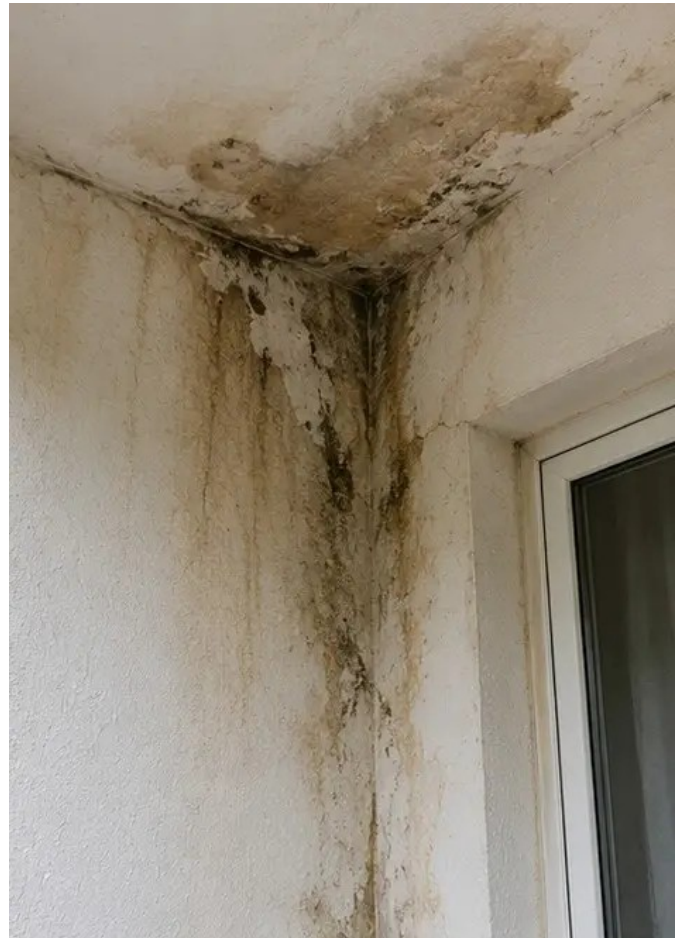
Photo #6 Water damage area identified and recorded
