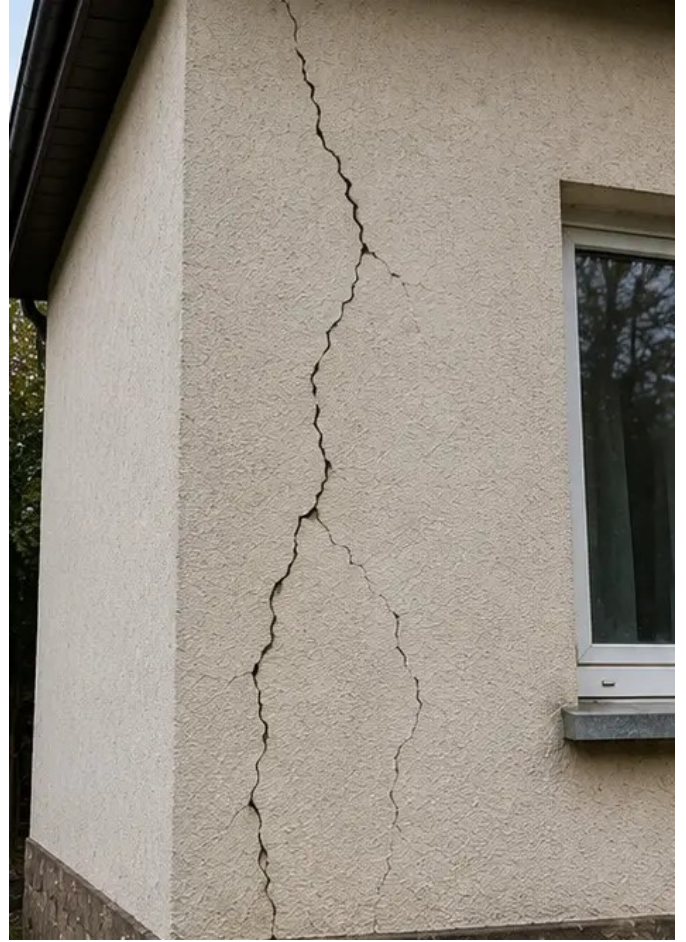
Photo #5 Structural wall crack documented during inspection
