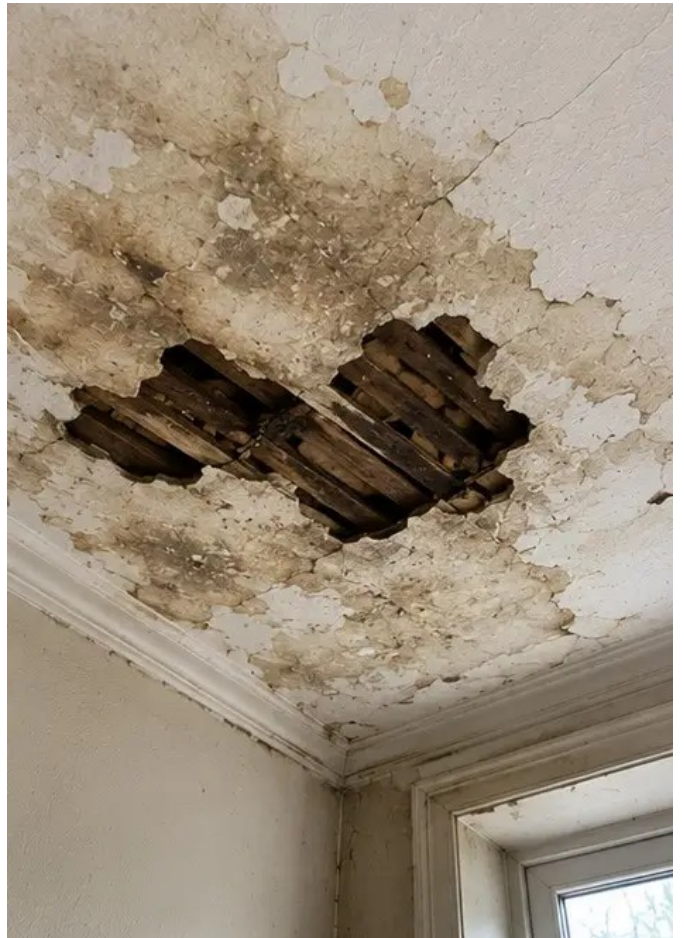
Photo #10 Ceiling damage identified and recorded
