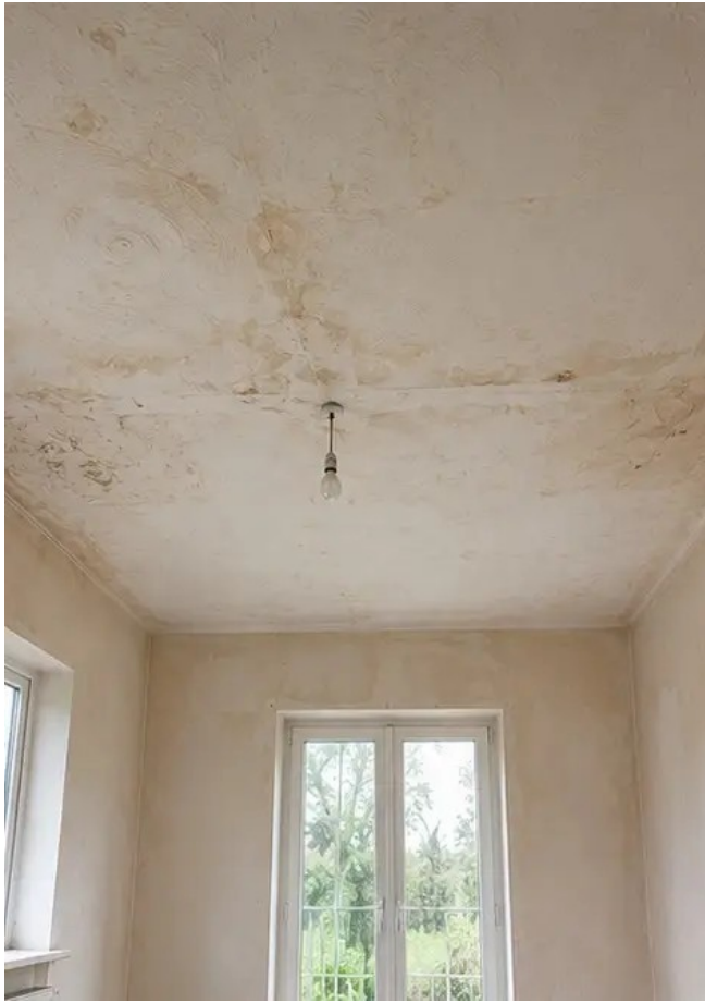
Photo #7 Ceiling condition before renovation
