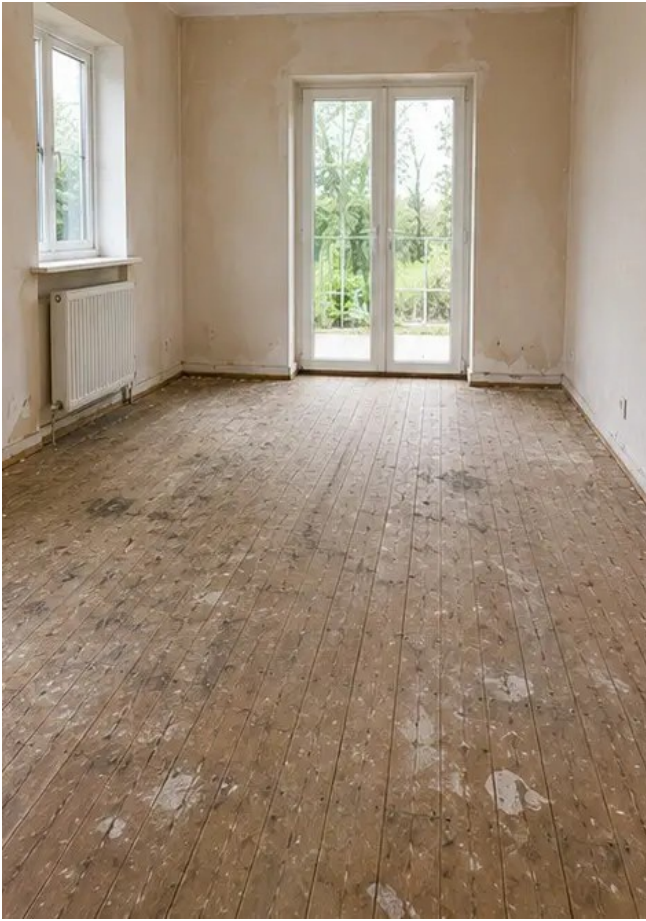
Photo #5 Flooring condition before replacement
