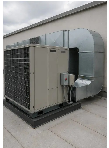
Photo #11. HVAC equipment condition assessed
