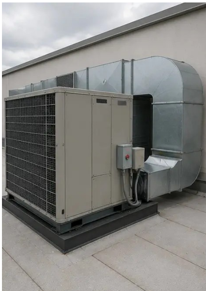
Photo #11. HVAC equipment condition assessed
