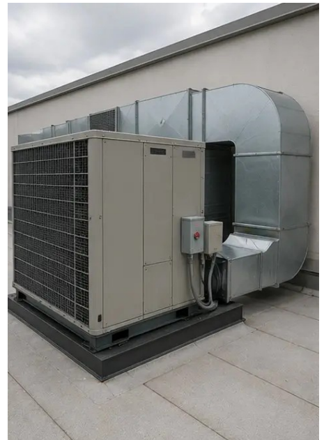
Photo #11. HVAC equipment condition assessed
