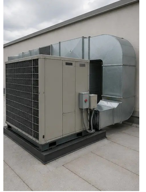
Photo #11. HVAC equipment condition assessed
