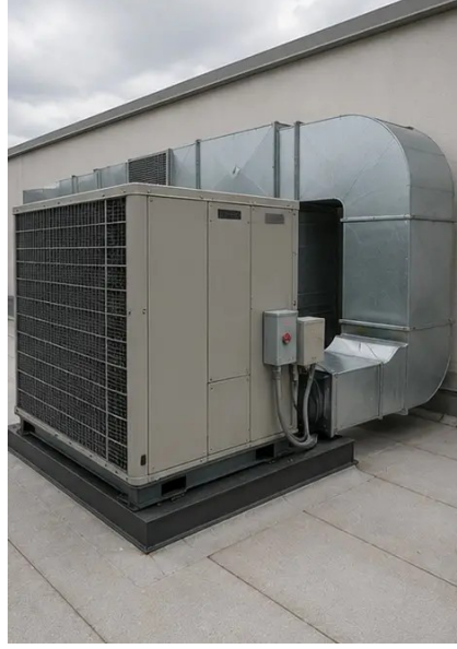
Photo #11. HVAC equipment condition assessed
