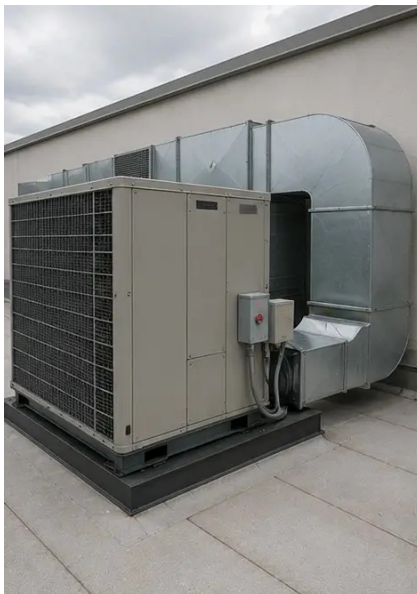
Photo #11. HVAC equipment condition assessed
