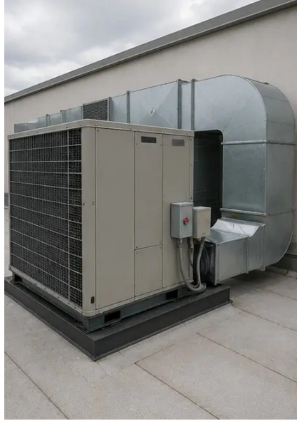
Photo #11. HVAC equipment condition assessed
